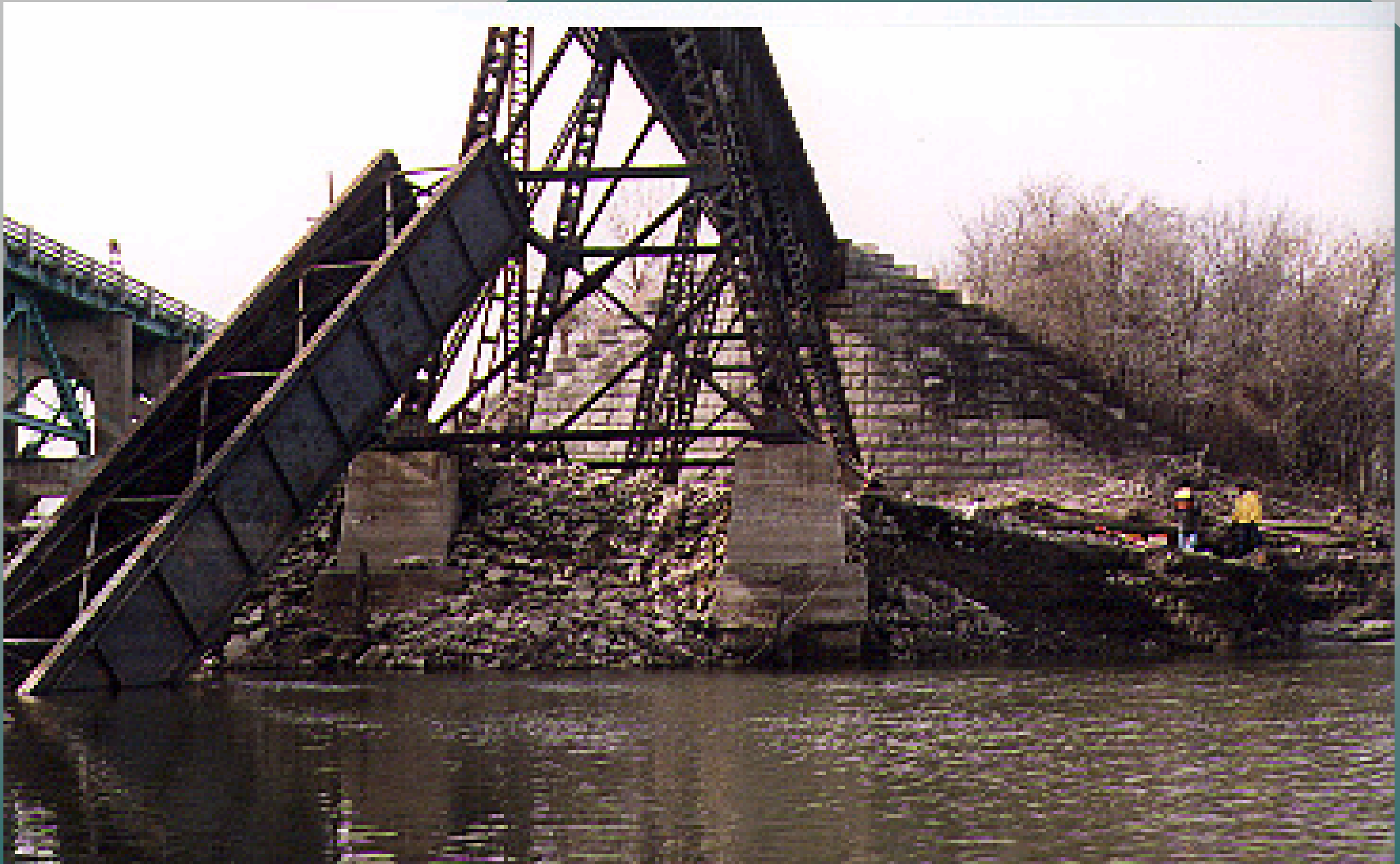
Bridge Failure Due to Scour, Glasgow, Missouri
