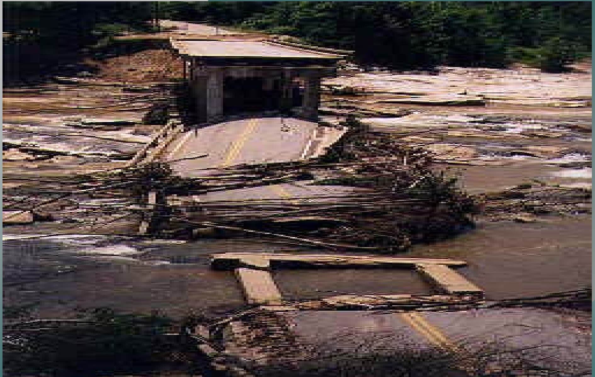
Bridge on the Enoree river in South Carolina which failed due to scour at the base of the piers caused by a turbulent horseshoe vortex system.
