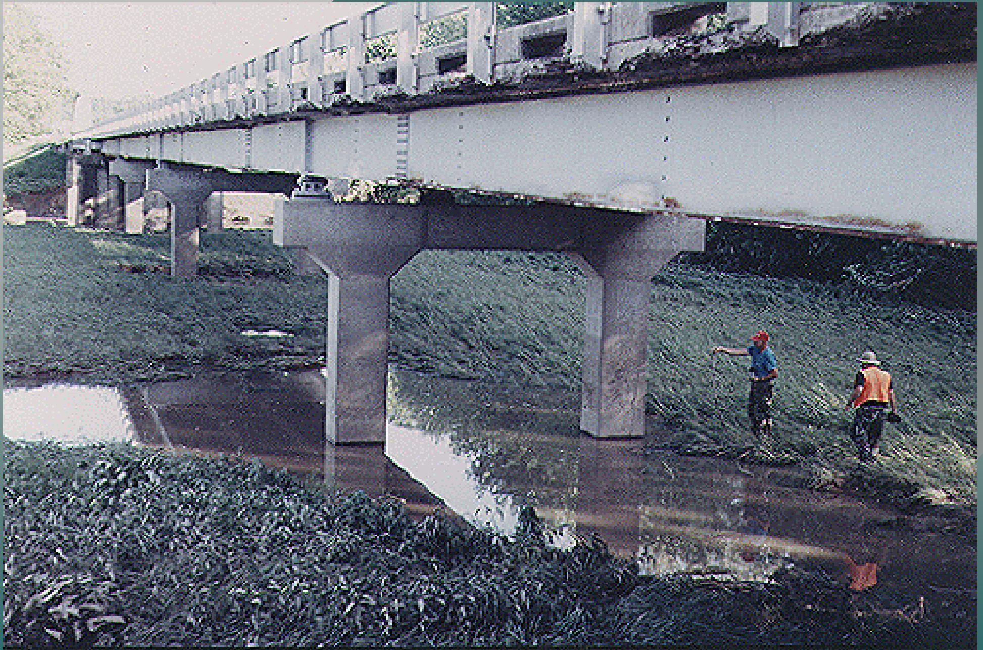
Contraction scour (somewhere) in Missouri during May and June of 1995.
